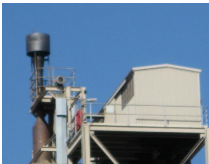
Figure 10: Flare stack used to flare off-gases during an incinerator trip
