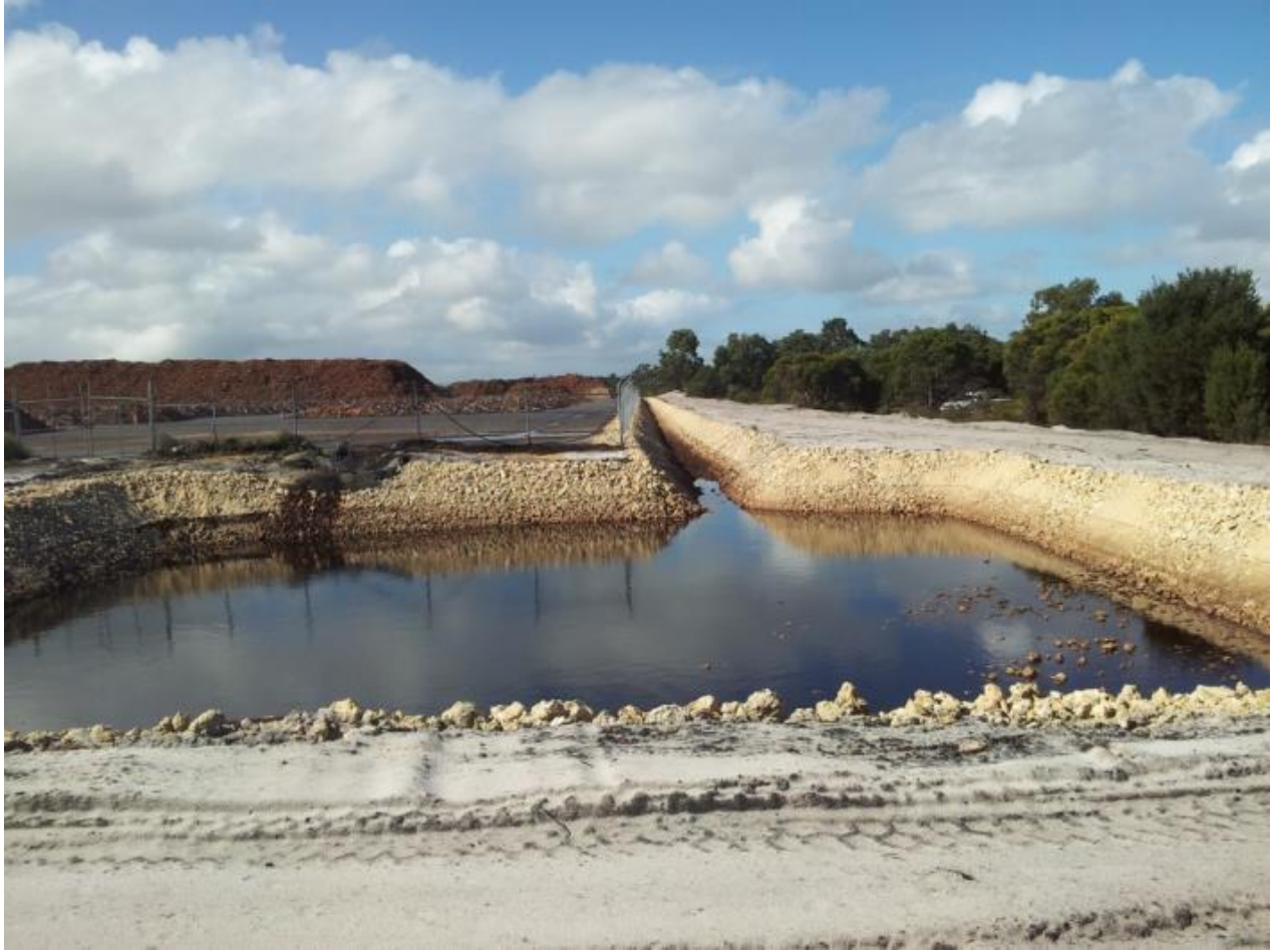
Figure 12: Infiltration drain and pond, which prevents erosion caused by stormwater runoff from the block pad
