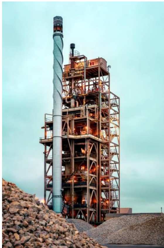
Figure 4: Charcoal Retorts: a source of noise from the Kemerton plant
